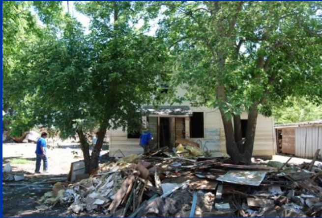
Volunteers clean up flood-damaged home. Photo courtesy Presbytery of East Iowa.
